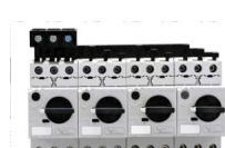
MMSs with bus bar connection
