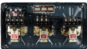
Interior View of MK1 SASD
