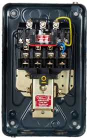
Interior View of MK1 DOL
