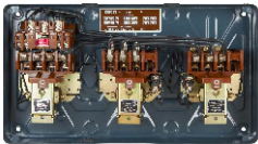
Interior View of MK2 SASD
